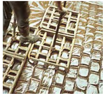
Figure 28 Plastic sheeting used to prevent concrete sticking to the mould – cobblestone texture
