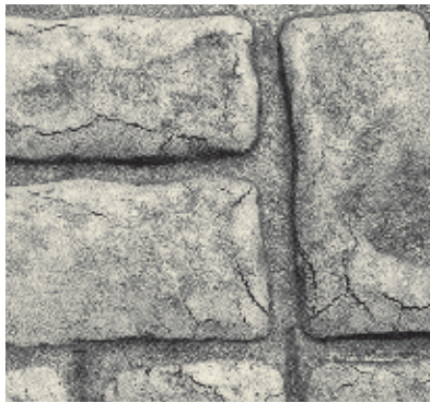
Figure 24 Crusting around edges of stamped pattern due to drying of the surface prior to stamping
