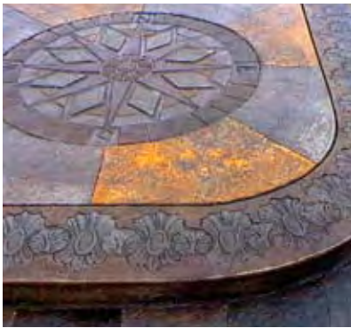
Figure 10 Mottled finish typical of chemically stained concrete (on stamped surface)
