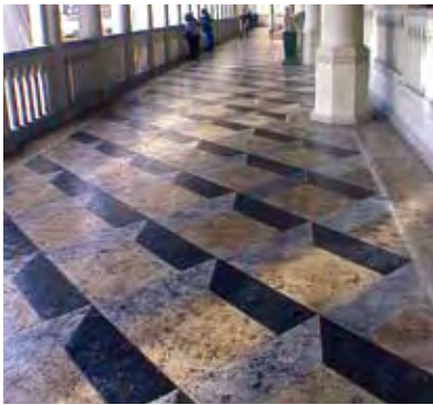
Figure 4 Surface coloured by chemical staining. Thin topping layer used to provide more consistent colours over large areas
