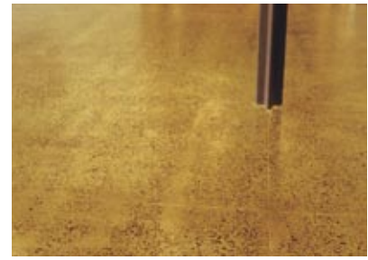
Figure 39 Sand streaks caused by dragging an immersion vibrator through a concrete topping
